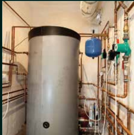
RAINWATER HARVESTING SYSTEM
