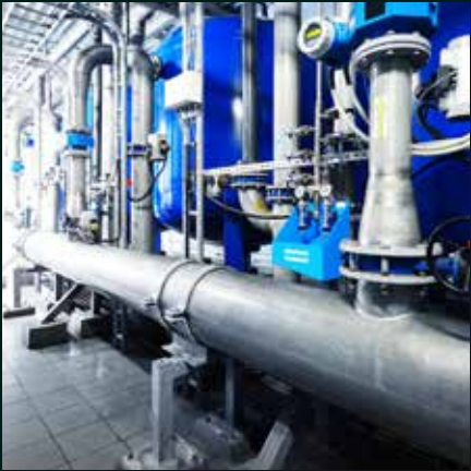
INDEPENDENT SEWAGE & WATER TREATMENT PLANT FOR EACH CLUSTER
