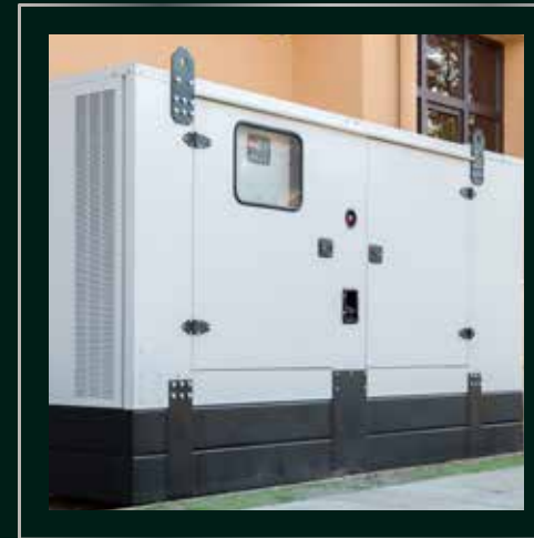
POWER BACKUP IN COMMON AREAS
