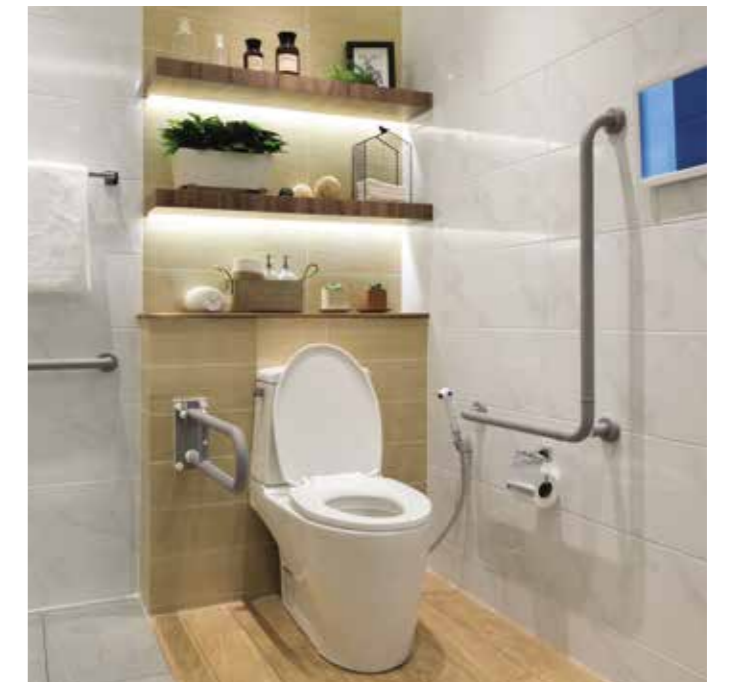
HAND RAILING IN ONE TOILET
